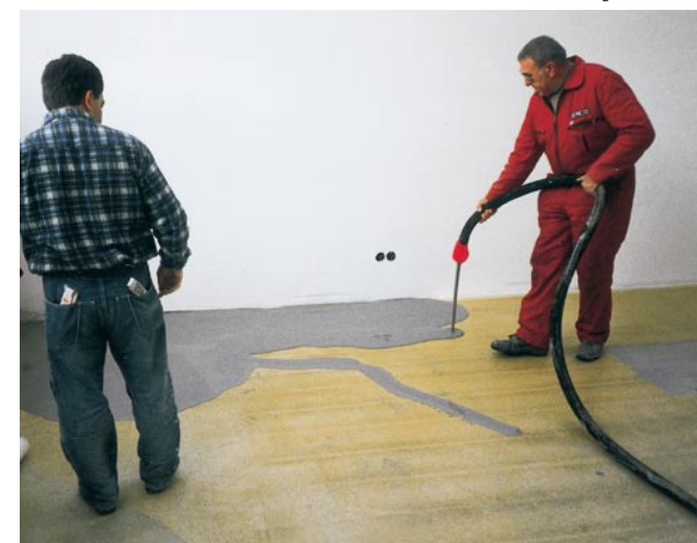
But even liquid cement filler can be worked (here e.g. with an S 5 EV TM in a production hall).
